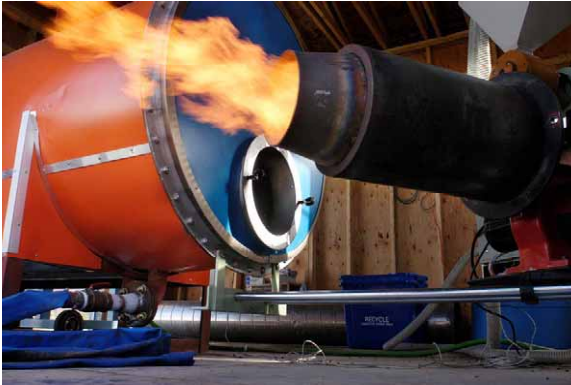
Figure 4. This is the hot water boiler housed in the boiler building at the Horticulture Research Farm. Hot water heated by the unit is used to heat high tunnels nearby. Here, the burner (right) has been pulled out of the boiler (left) for demonstration purposes to show the flame while burning plastic fuel.
